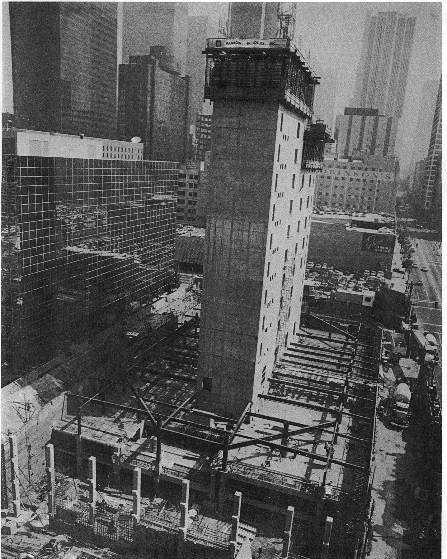
Jump formed concrete core at Grand Financial Plaza, downtown Los Angeles, illustrates unique steel and concrete composite structural system for seismic zone 4.
